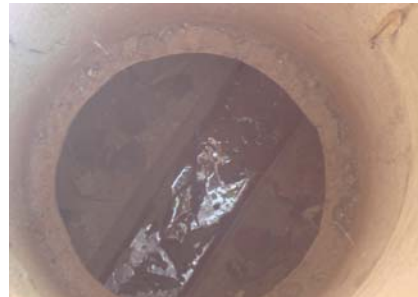
Sewage flowing in existing Manhole
