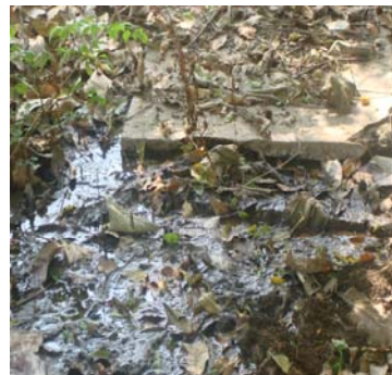
Sewage overflowing from the manhole
