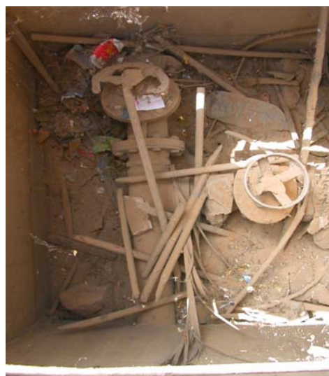
Existing Water supply valve chamber
