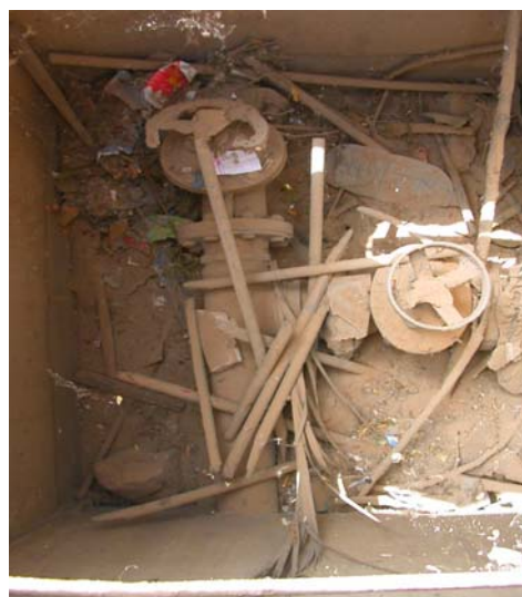
Existing Water supply valve chamber
