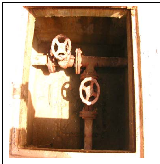
Corroded valve chamber
